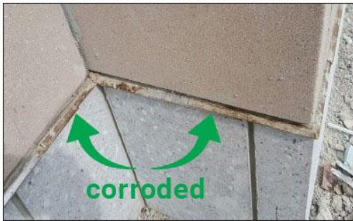
Corroded imported stainless steel drip edge not held to DFARS standards.
